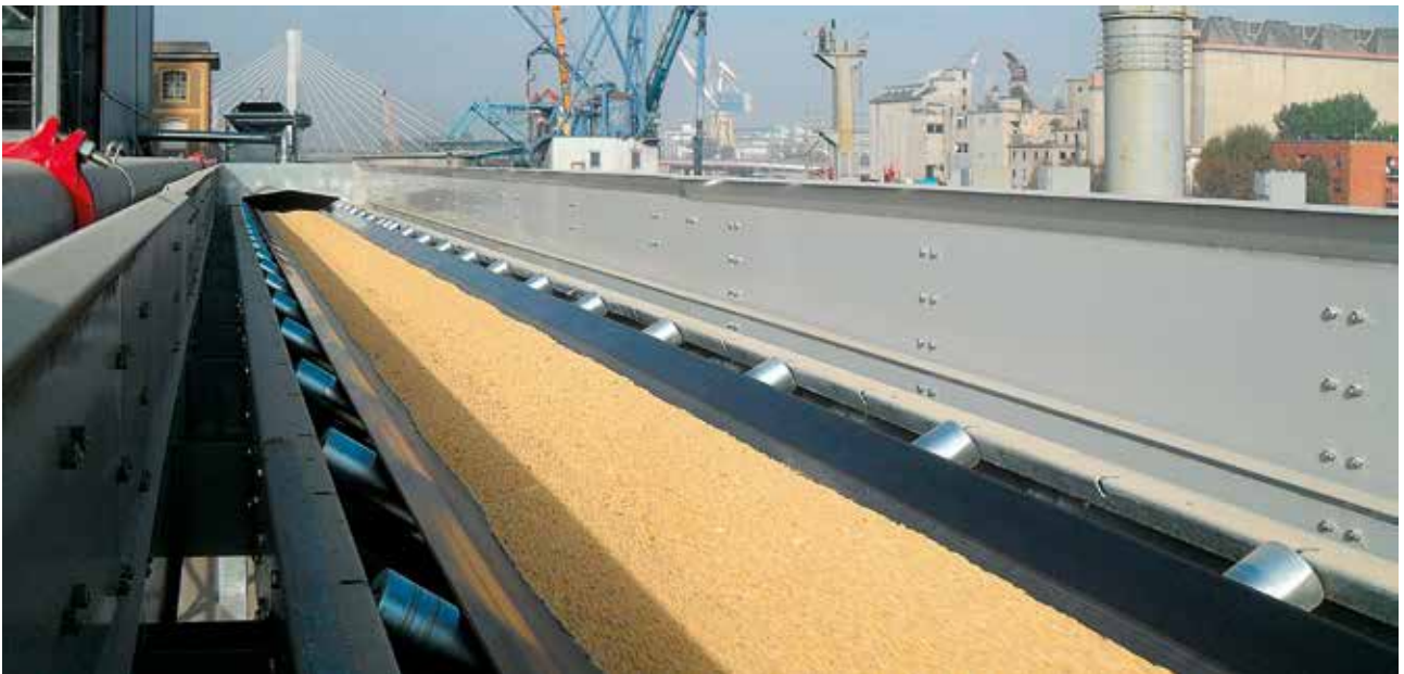
Belt conveyor MXB 63.120 with capacity of 1000 t/h
