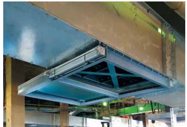
Detailed view of unloading shutter
